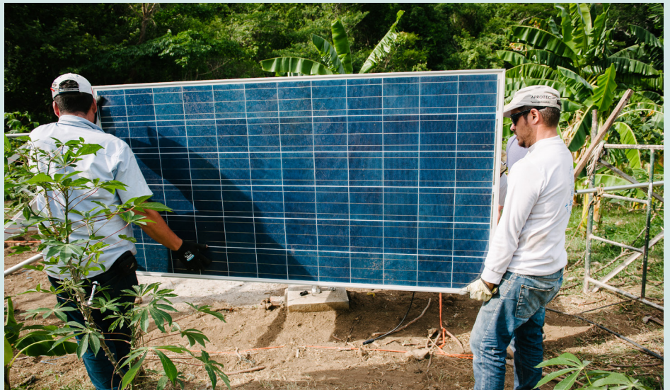
Installation of solar panels at Sabana Crespo health facility, Colombia. Photo: Alex Adams Photography
